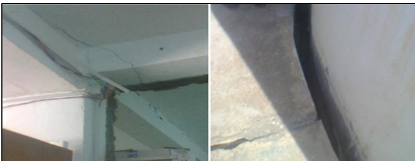
Fig. 3. Effects of landslides on the interior of collective dwellings (Source: Authors, 2021)
