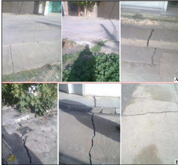
Fig. 5. Effects of landslides on streets (A: Rue Louanas, B: Rue Djebri Aissa) (Source: Authors, 2021)
