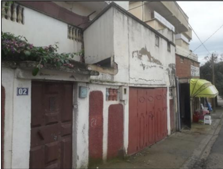
Fig. 10. A house affected by landslides (Source: Authors, 2021)
