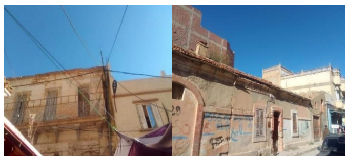
Fig. 2. Degradation of the colonial building of the old center of the city of Ain-Beida (Source: author, 2022)
