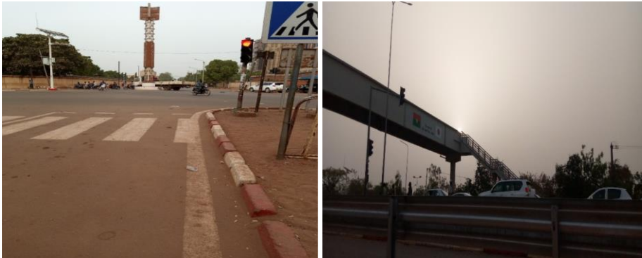
Fig. 5. Pedestrian crossings built but not used (Soma et al., field observation, June 2022)
