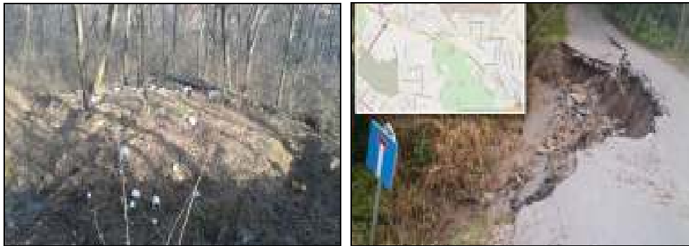
Figures 5 and 6. Landslide and “wild” landfill (left, 50m away from the boundary of NM) (Samardžić I., 2016.), ruined infrastructure (right), (www.telegraf.rs from 2014, corner of Ramska Street and Volgina Street)
